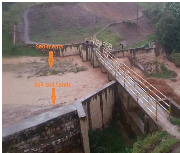
Figure 6 Impact of heavy rain on hydropower plant
