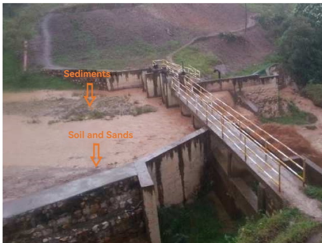
Figure 6 Impact of heavy rain on hydropower plant
