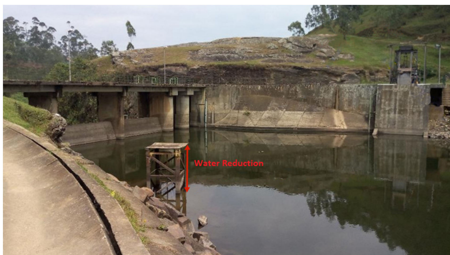
Figure 7 Impact of long dry season on hydropower plant
